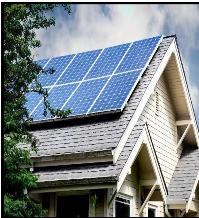
Roof solar panels
